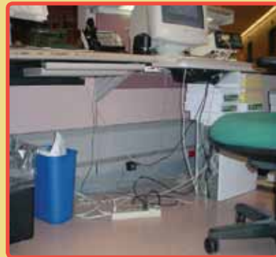
Figure 9.6. Loose cords at nursing workstation
