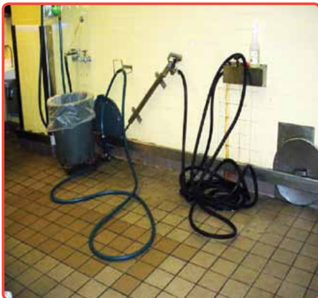
Figure 9.5. Uncoiled hose in a walkway
