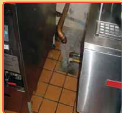
Figure 2.3. Pipe splashing water onto the floor around a drain
