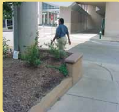
Figure 2.5c. Corrected drainpipe. Water was diverted underground to the sewer pipe, and spout no longer directed onto sidewalk
